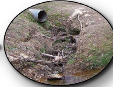
Pipe Outfall to Water Body (Volume and Velocity Cause Erosion and Degradation)
